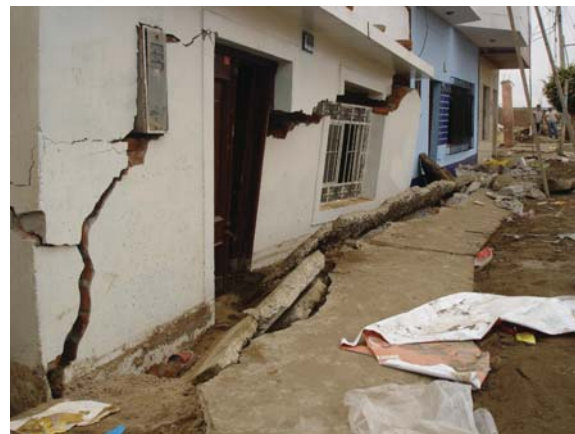
Figure 6. The situation was better in Peru where reinforced concrete was used. However note that 45 degree earthquake cracks from shear forces can be seen on masonry structures.
