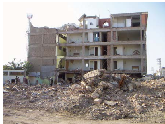
Figure 7. Brick walls collapsed while the infrastructure held up because the concrete structure was sturdy and well designed. However in long spans (on the right), because of poor wall retention all the bricks collapsed.
